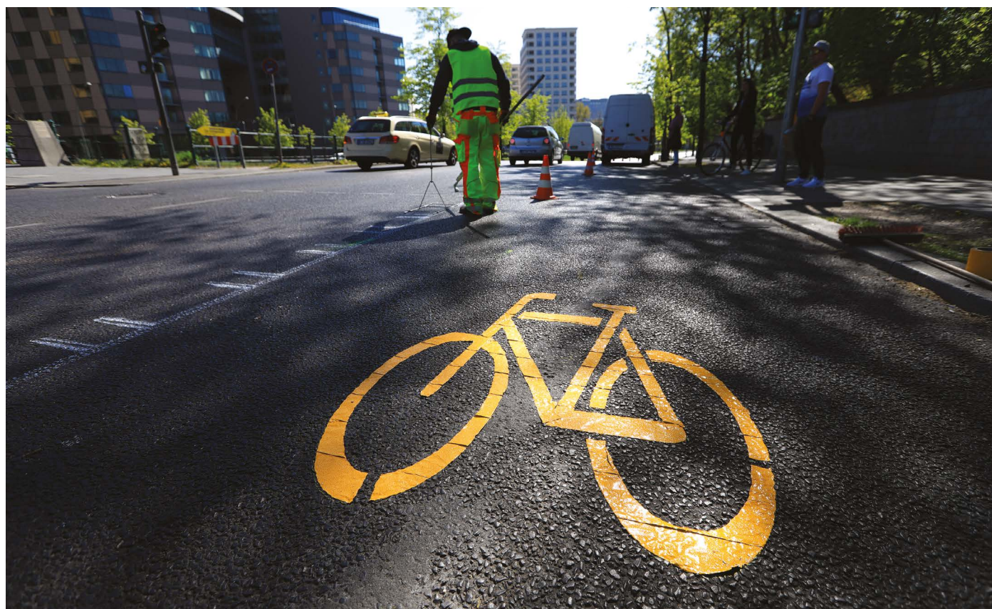
Pop-up cycle lanes were installed across Germany during the COVID-19 pandemic to aid social distancing.
