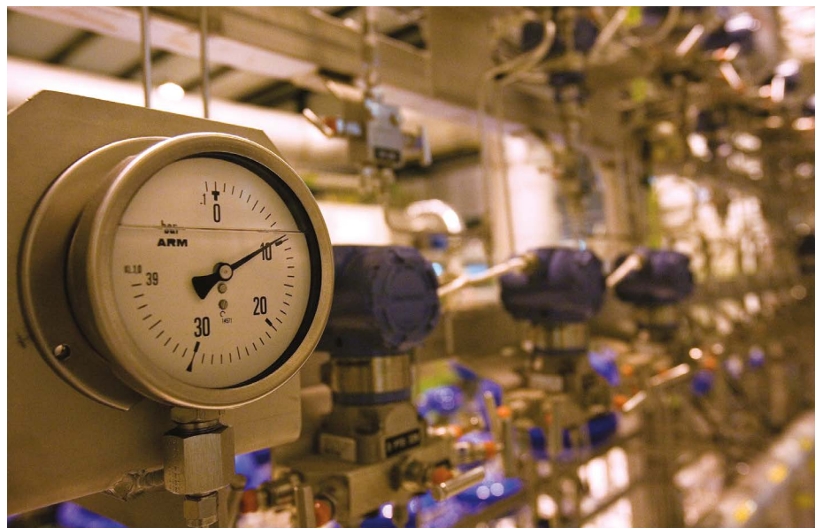
Cryogenics account for more than half of the LHC's electricity consumption.
